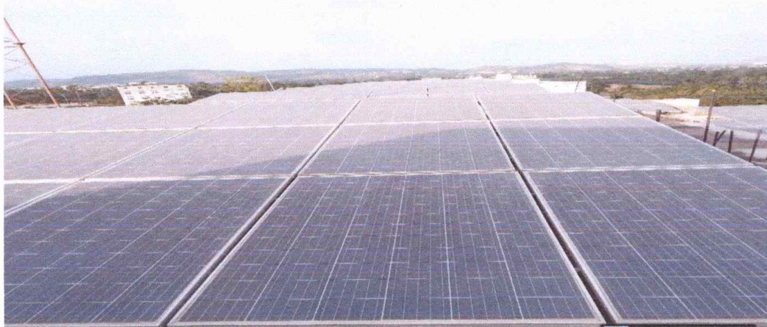
FIG: 6 Installed solar panels that consist the capacity of 60 KW Each
